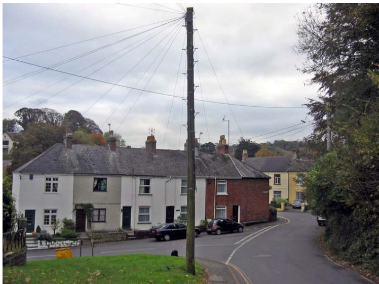
Wiring on Underwood Road
