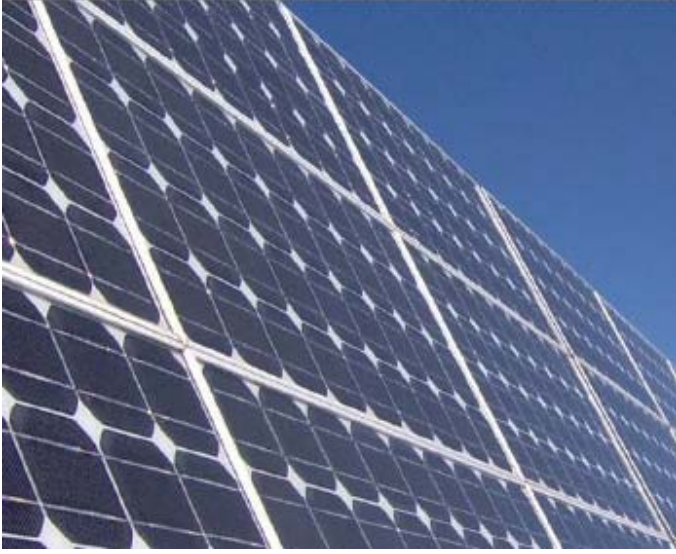
Mono-crystalline PV Panels
